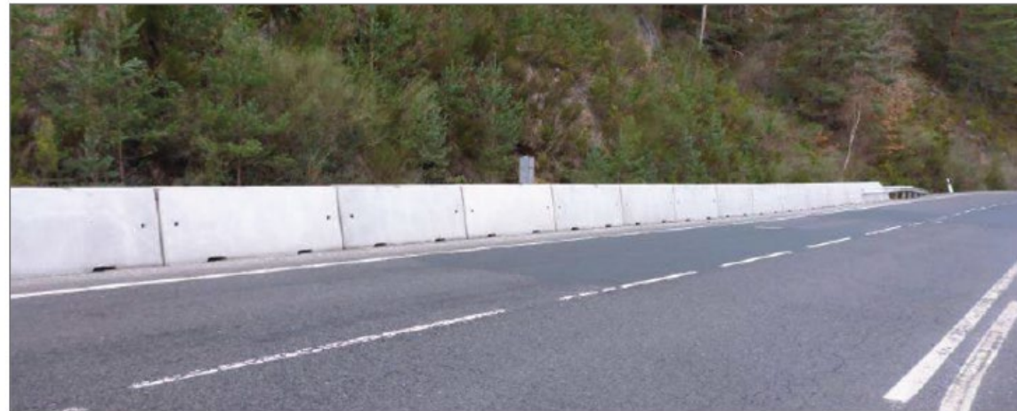
Precast concrete New Jersey barriers
